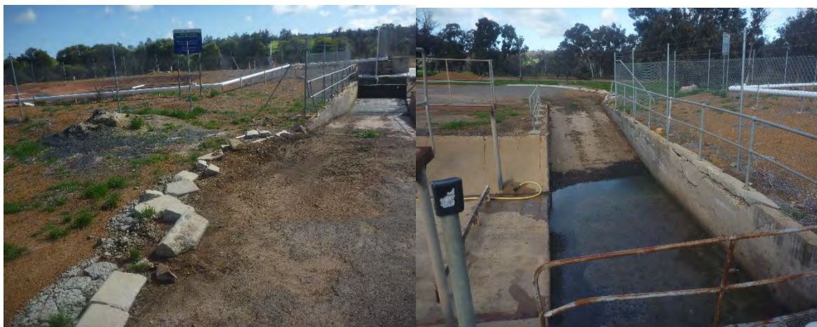
Photo 9 & 10 maintenance issues Kojonup truck wash.
